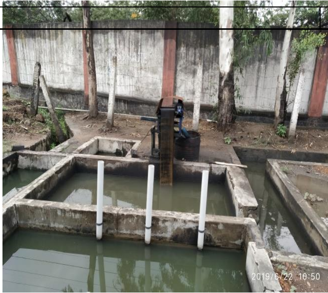
Aeration tank and Oil skimmer
